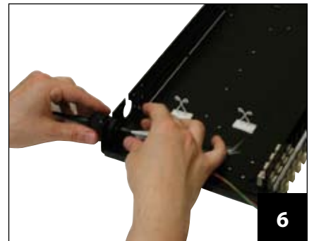
6 Install the fibre cable assembly in to the fibre patch panel.
